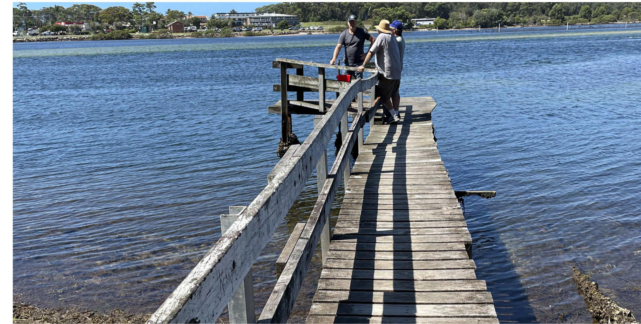
Character, charm and suitability for the environment of existing structures will inform new ones, including the rational geometries.
